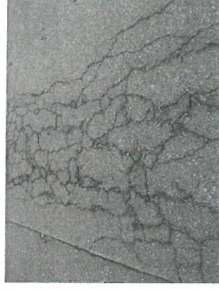
Alligator Cracked Roadway.
