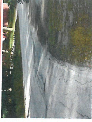
Roadway & Driveway Damage.
