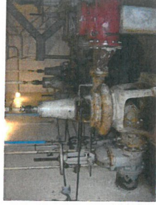
Pump motors to be replaced
