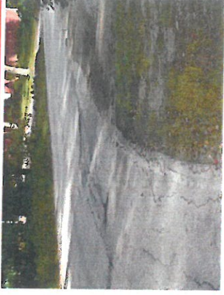
Roadway & Driveway Damage.
