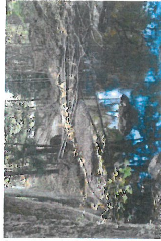
Bank erosion from high velocity flows through current structure..
