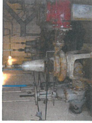
Pump motors to be replaced
