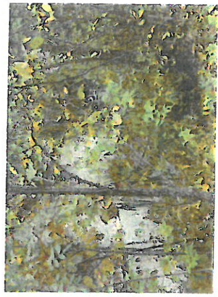
Deteriorating CMP Pipe
