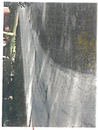
Roadway & Driveway Damage.
