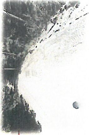
Greens Pond Rd – note erosion to the right
