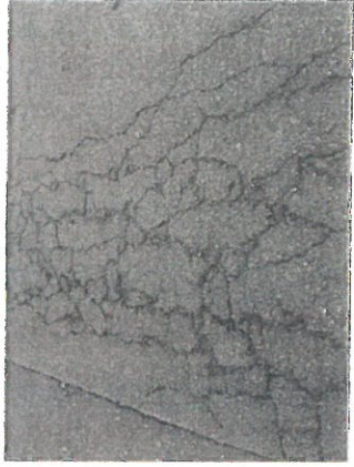
Alligator Cracked Roadway.
