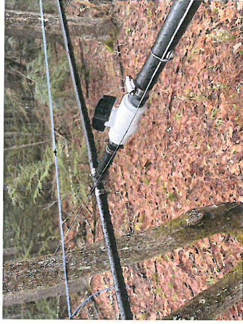
Ball Valve to close off sections for leak detection
