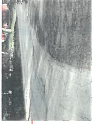
Roadway & Driveway Damage.
