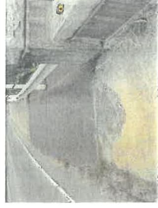
Failed sidewalk on DW Hwy
