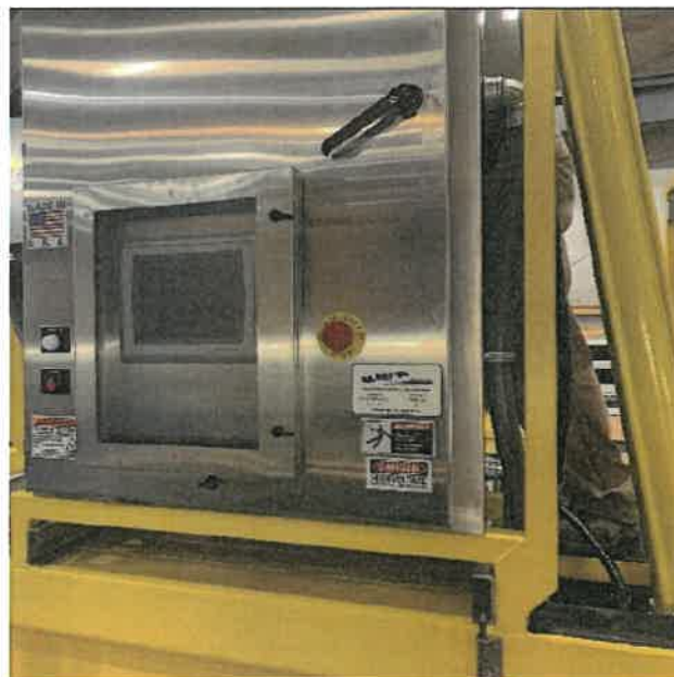
Control Panel Location on Dolly which remains outside the bays
