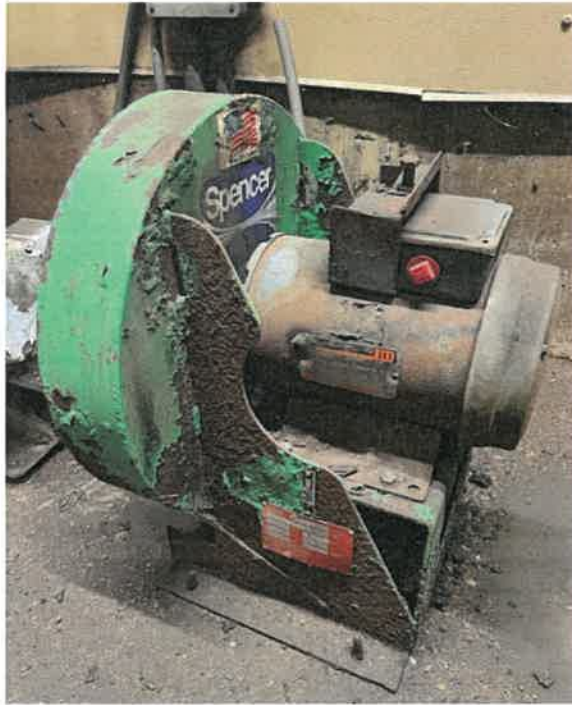
Existing Compost Blower
