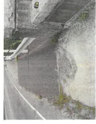
Failed sidewalk on DW Hwy
