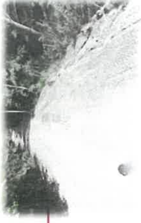
Greens Pond Rd – note erosion to the right
