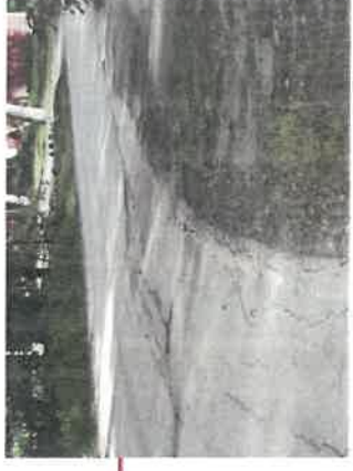
Roadway & Driveway Damage.
