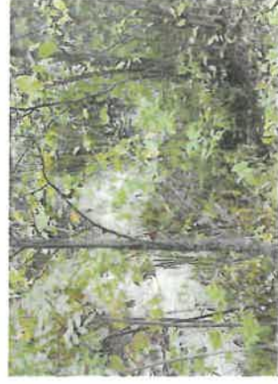
Deteriorating CMP Pipe
