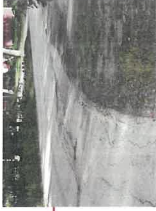
Roadway & Driveway Damage.
