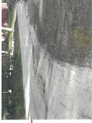
Roadway & Driveway Damage.
