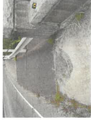
Failed sidewalk on DW Hwy
