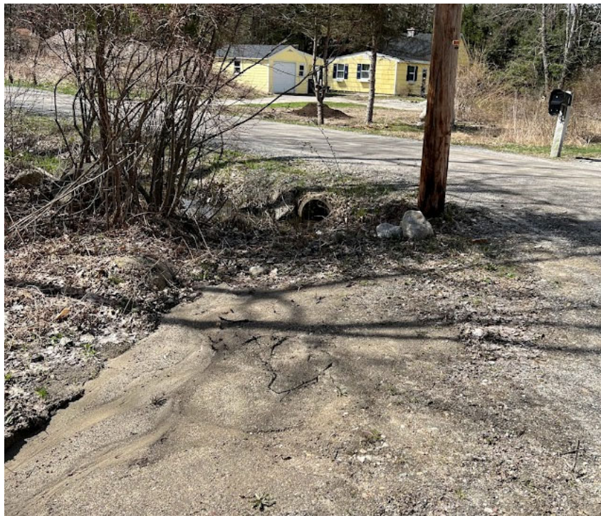
Photo 7. Sediment washout area at corner of Mayhew & Rennie.
