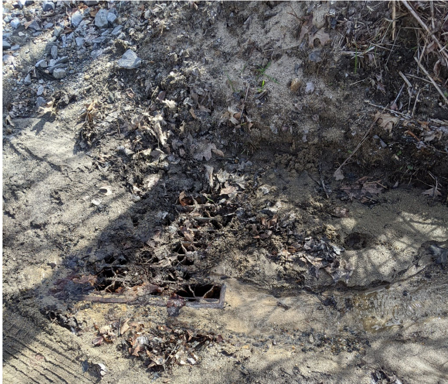
Photo 9. Silted-over catch basin at corner of Rennie & Carter (note: Carter is paved; Rennie is unpaved).
