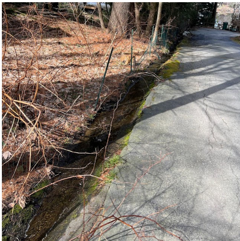
Photo 6. Overland flow draining from Shore Drive to Baboosic Lake through property at 20 Shore Drive.
