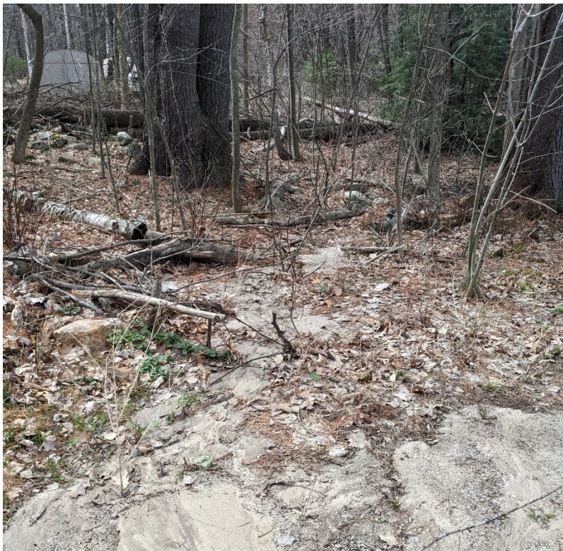
Photo 5. Town property on Mayhew Road. Note the sediment washout onto the property from the adjacent road.
