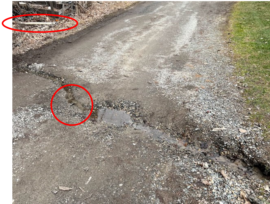
Photo 10. Roadway washout area on Baxter Lane. Note: crushed remnants of former 6" PVC culvert still visible in roadway where indicated. Residents removed half of piping; visible adjacent to roadway as indicated.
